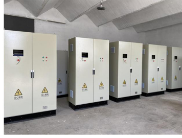
Energy storage system
